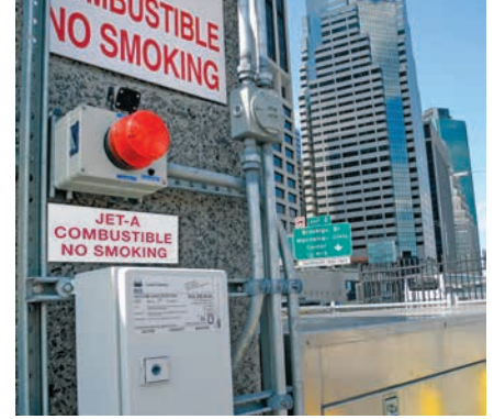
The explosion-protected vacuum leak detector next to the pumping station
