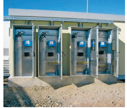
Positive pressure leak detectors in protective housings
