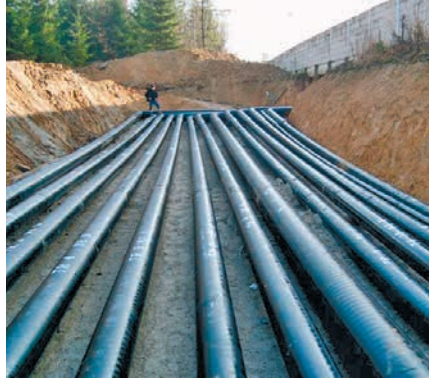
Routing crossing the motorway below
