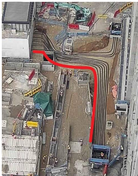
Figure 1 Uninterrupted Pipe Run
