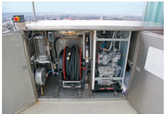
Tanking cabinet with Jet A-1
