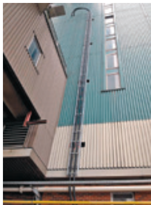
Riser line on the flue gas scrubber plant
