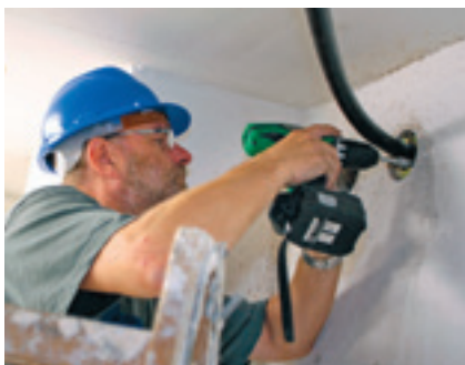
Applying a fire-retarding seal to the FLEXWELL® Safety Pipe with an approved specification fire safety wall duct.
