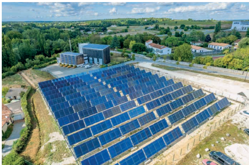
Figure 1. A solar thermal power station of 1,800 m 2 supplies the heating network of the city of Pons
